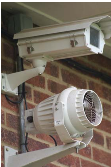
(Rayne – CCTV Equipment – Village Hall)
